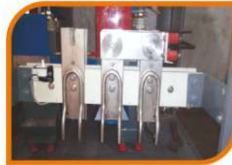
Furnace Selector Switch
